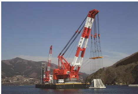
Construction work on the breakwater in Ofunato Port (Photo: Kamaishi Port Office)
