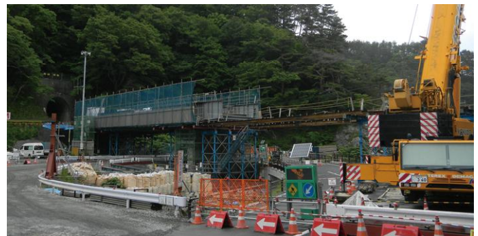
Work on the land bridge between Tanohata and Shimanokoshi Stations. ※The substructure is completed, and work on installing the beams has begun.
