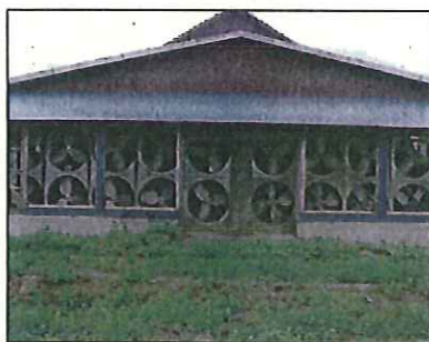
↑牛舎壁面の換気扇
