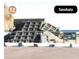
12 Remnants of Earthquake Aketo Coastal Sea Wall Tanohata
